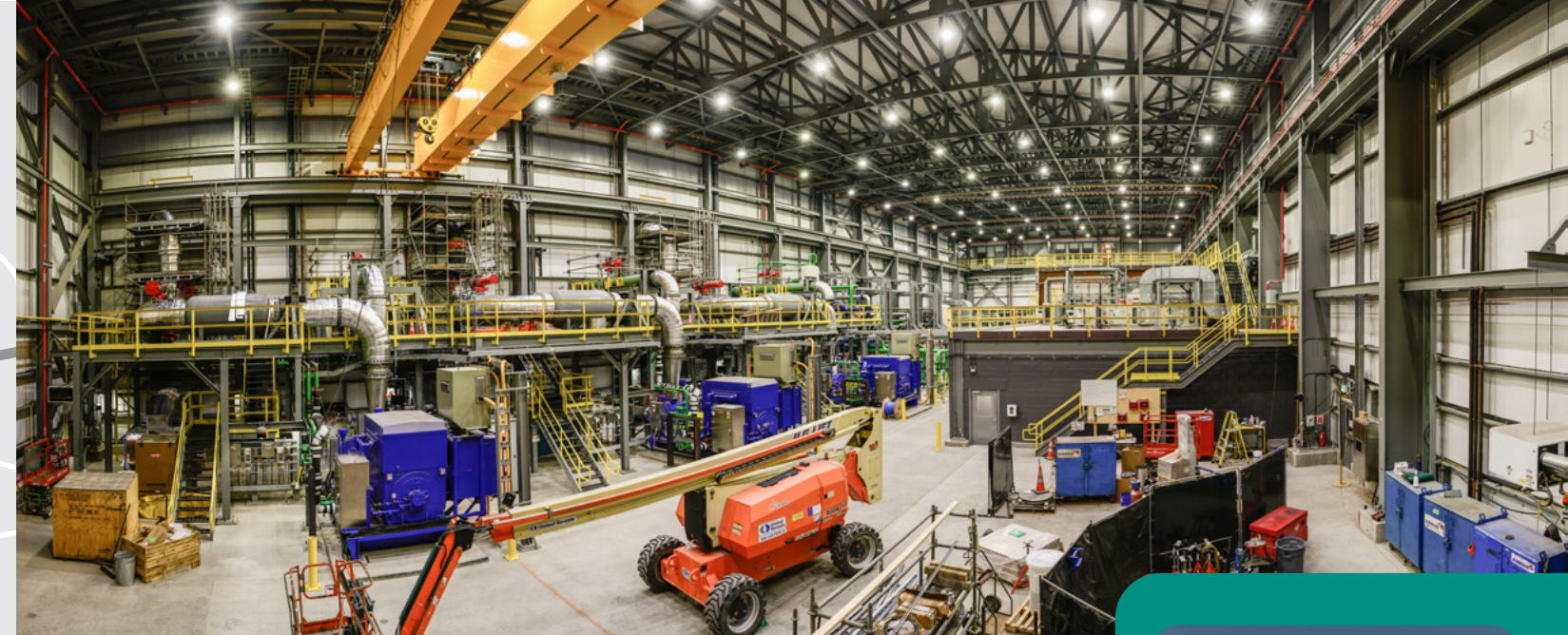
New surface utilities building is designed to modernize utilities infrastructure for the Smelter.
