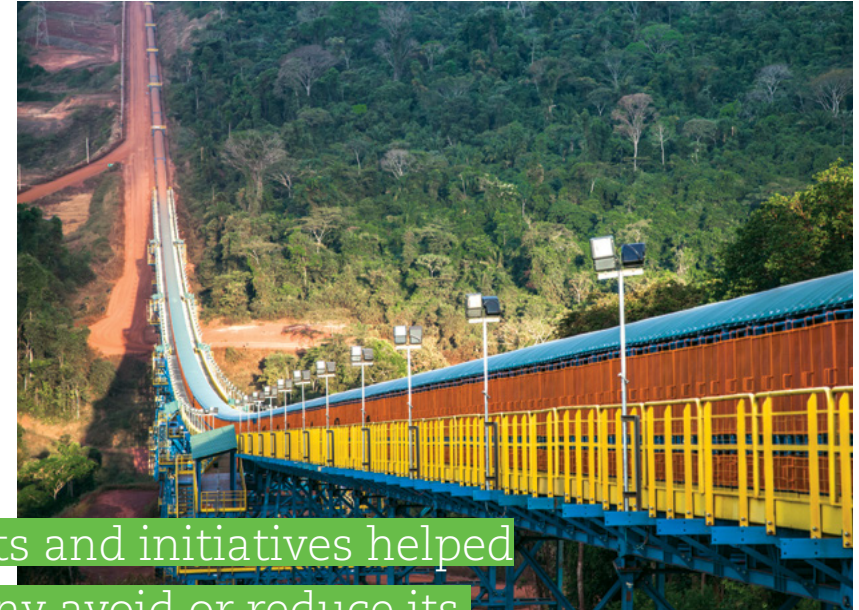
S11D Eliezer Batista Complex Long Distance Belt Conveyor, in Canaã dos Carajás (PA), one of Vale's initiatives to reduce emissions Photo: Ricardo Teles
