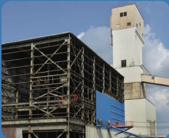
Asbestos cladding was removed from the Dewatering Area of the Mill and new inner siding is in progress.
