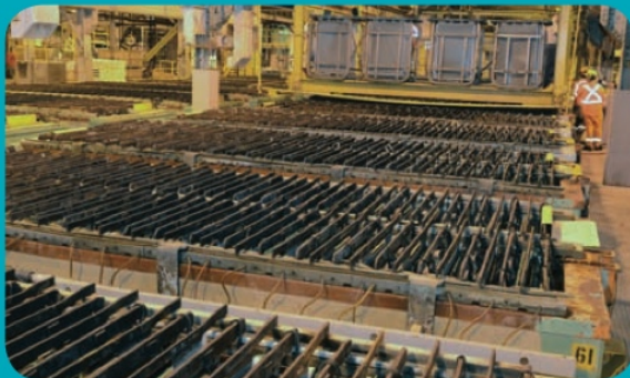
The Refinery Tankhouse is where anodes from the Smelter are dissolved, resulting in the nickel migrating to cathode sheets or mandrels (for Rounds production).
