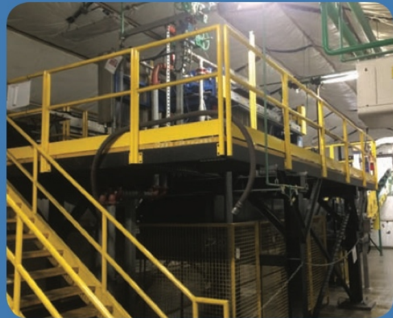
A temporary copper filter press was installed behind the Mill in order to free up the Dewatering Area for demolition and construction.
