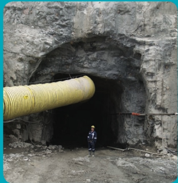
Birchtree Mine is the only mine in Manitoba Operations which you can enter through a portal (shown under construction) rather than down a shaft.
